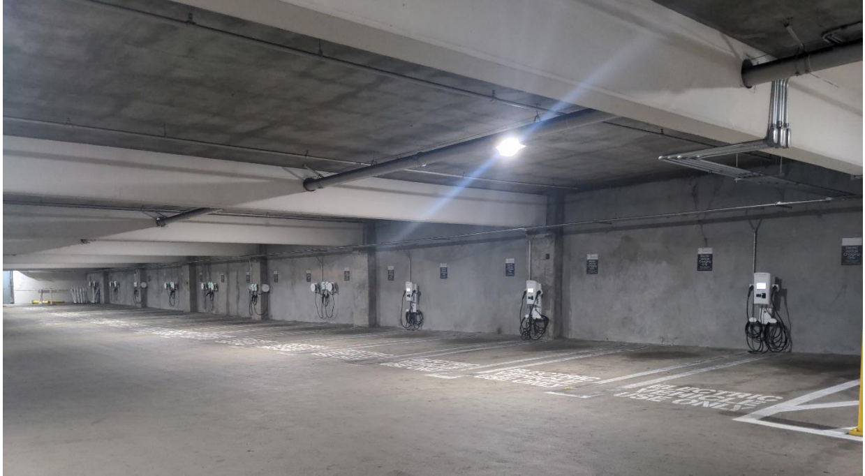
Glendale Marketplace Parking Structure EV Charging Stations
