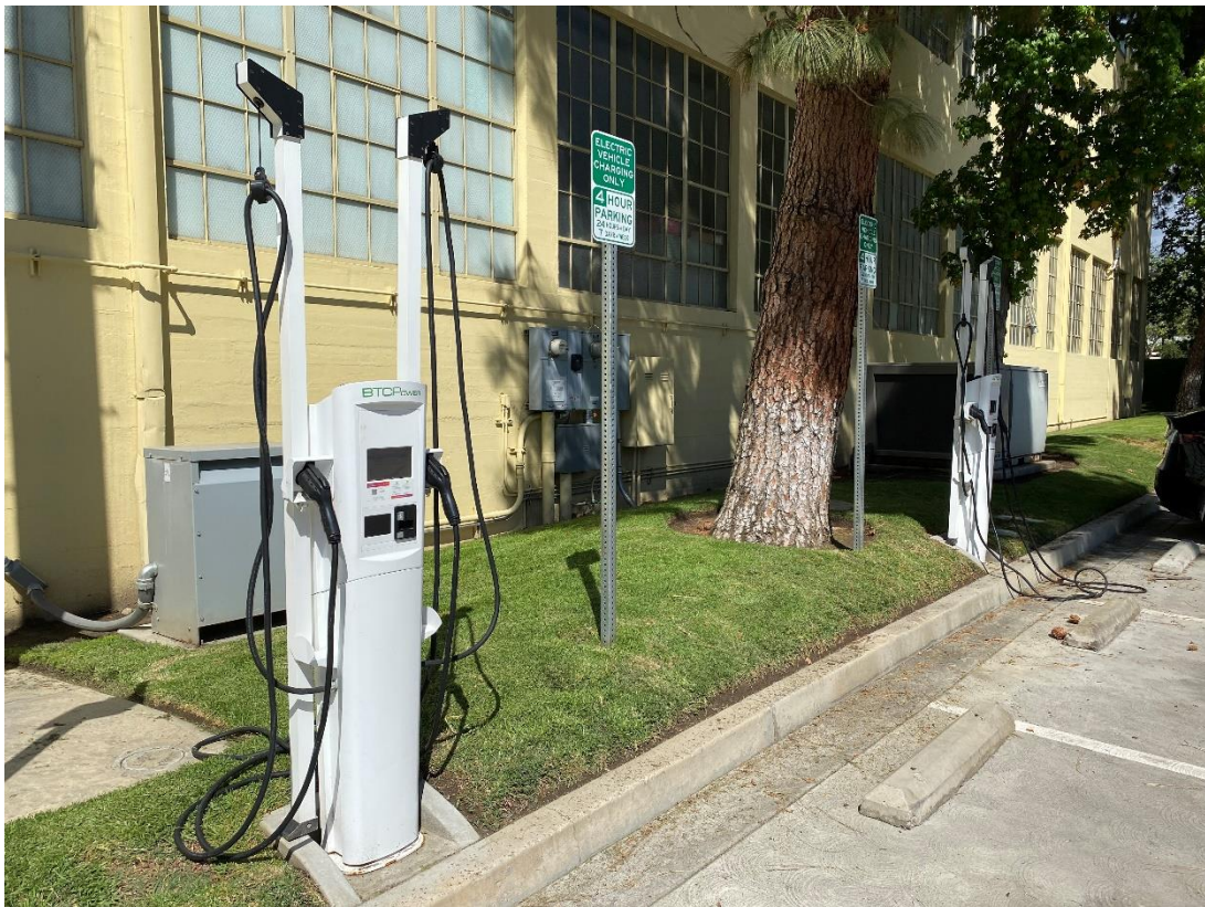
Glendale City Hall EV Charging Stations
